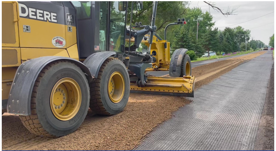
MCRC’s Poseyville Rd. rehabilitation project using geogrid geosynthetic material to enhance road base.
