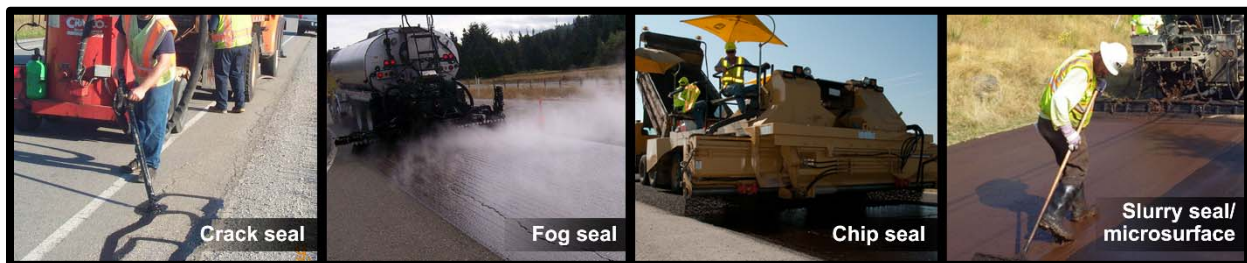
Figure 5: Examples of capital preventive maintenance treatments—(from left) crack seal, fog seal, chip seal, and slurry seal/microsurface.
